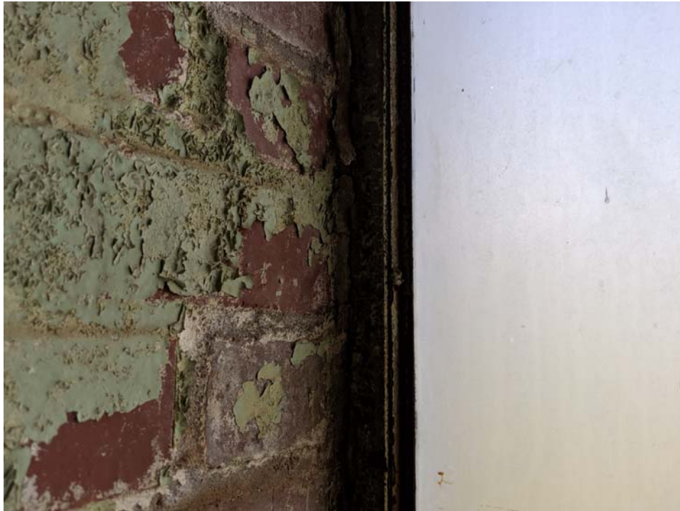
Asbestos containing window caulk between window sash and brick.
